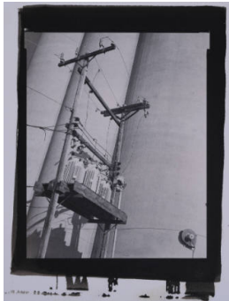
Title: Transformers at Grain Elevator Date: 1996 Primary Maker: Richard S. Sullivan Medium: Ziatype
